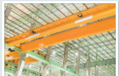
Overhead traveling crane
