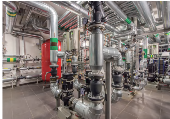
Municipal heating system
