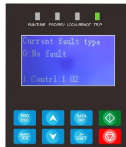
Faulty state displayed
