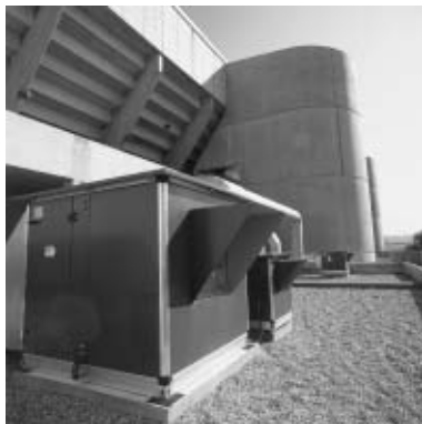
Air conditioning application
