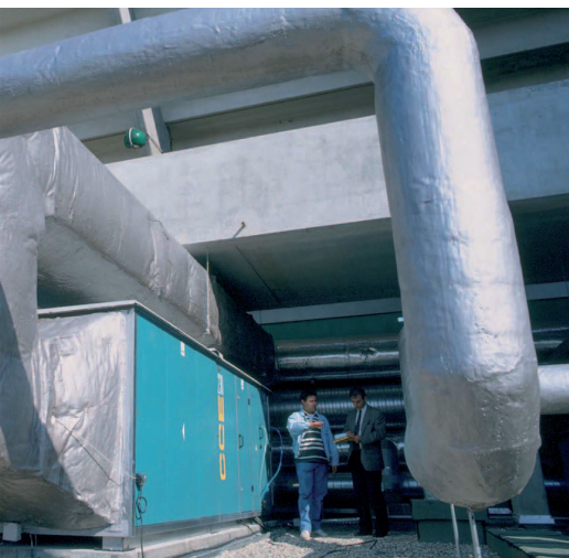
Circulating pumps for building management
