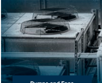
Pumps and Fans
