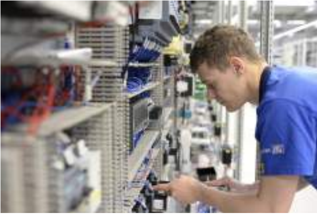
WKC - Control cabinet wiring
