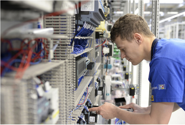
WKC - Control cabinet wiring
